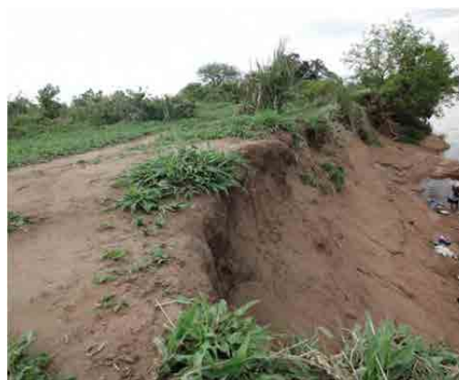
Photo 8-2 Bank Erosion of the Ruo River
