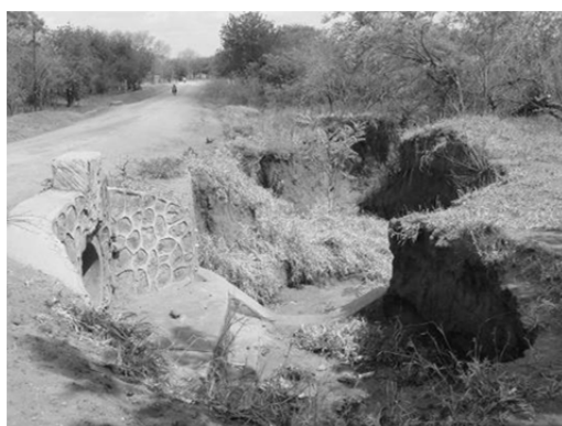
Scoured Drains at downstream side
