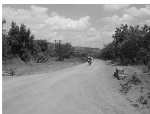
Gullies/ditches on the road sides
