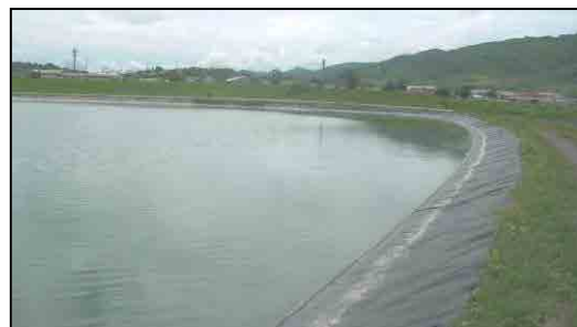
Photo 2 Treatment Facility (Settling Pond for Treatment)
