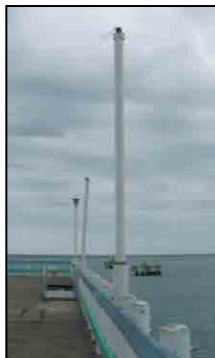
Photo 20 Broken Electric Lamp
