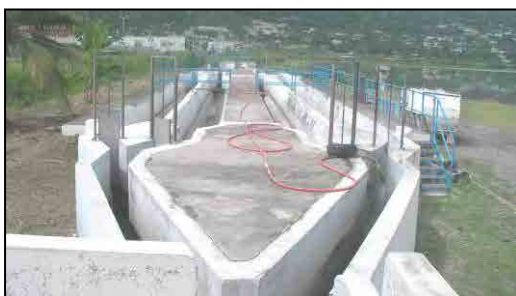
Photo 1 Treatment Facility (Sewage Inlet)
