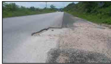
Photo 8 Road Damage (Damage to Road Shoulder)
