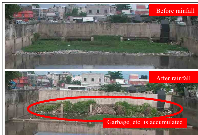
Photo 13 Conditions of Culvert Inlet Before and After Rainfall
