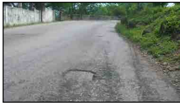
Photo 7 Road Damage (Pothole)
