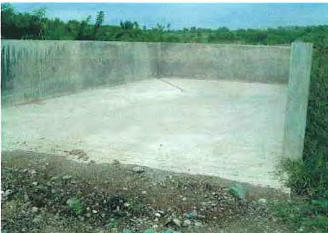
A overall view of manure burn (silo)
