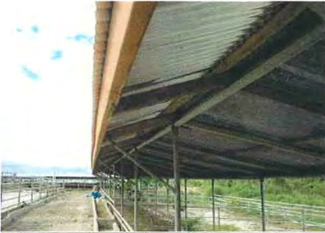
A wide view of re-roofing portion with painted frame with orange color
