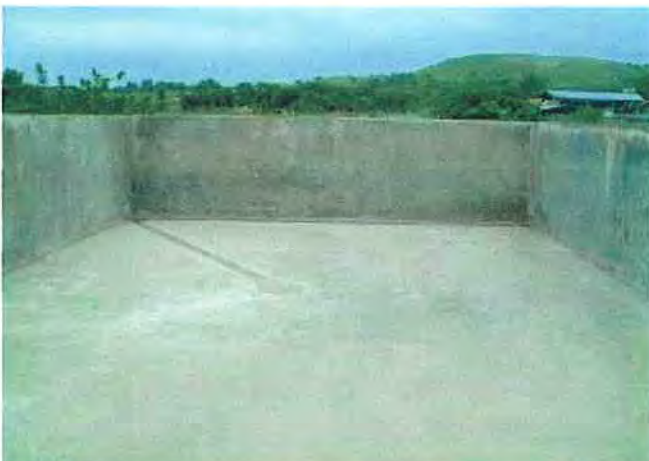
Alteration of floor, small catch basin and drainage for effluence from silage
