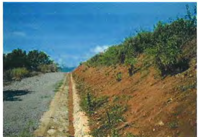
A rip rap canal was installed and the angle of the slope was adjusted to 45 degrees to prevent land slide
