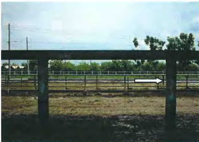
The arrow shows the portion where a steel pipe added
