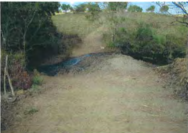
Heavy damaged slope to the river
