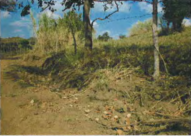
Collapsed portion in the middle of the road
