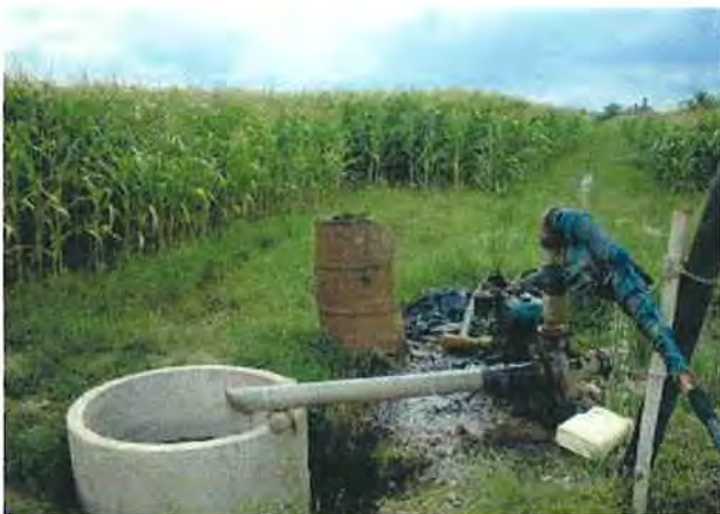
A well was newly installed beside the shed by cooperative members for buffalo management and pastureland irrigation
