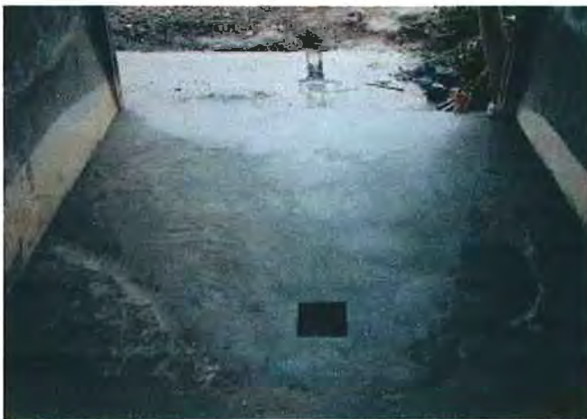
Re-cemented floor after installation of drain pipe, and catch basin is left on the floor
