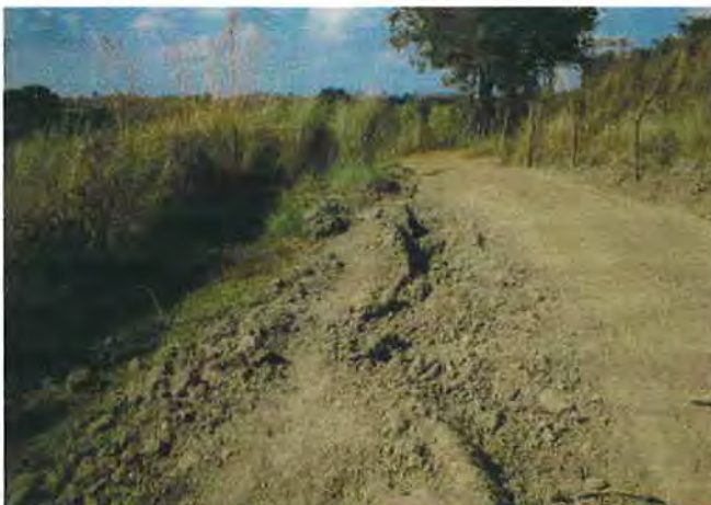
Shoulder is eroded by rain water from the left
