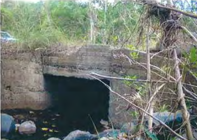
A box type culvert was placed at the starting point of the access road rehabilitated. Displacement of this culvert was not enough to drain water during rainy season.
