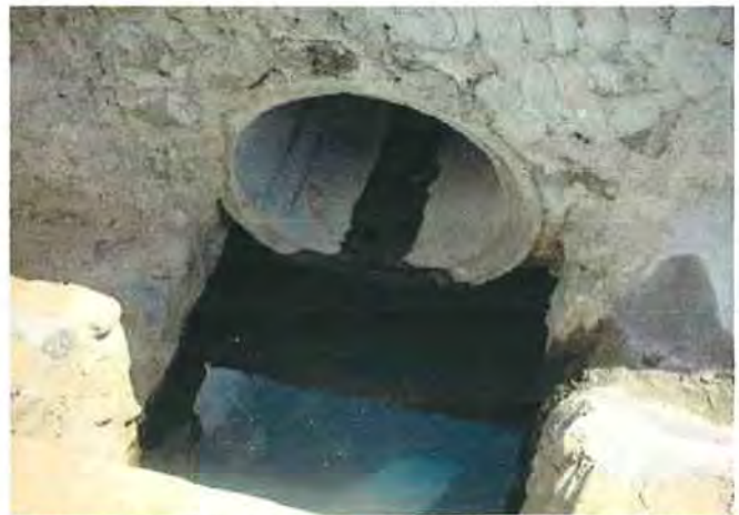
A big size of culvert with catch basin was prepared for draining water (Inlet)
