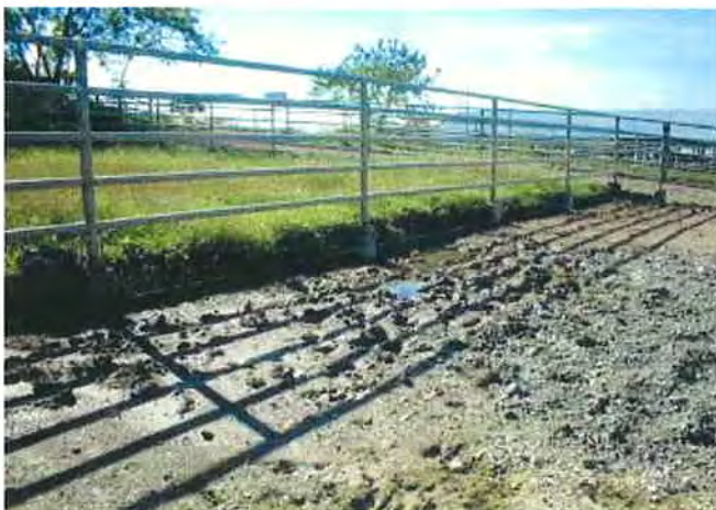
A condition of after raining
