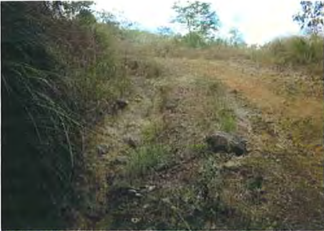
An Eroded portion in curve
