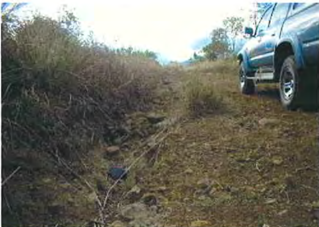
An eroded portion on the shoulder
