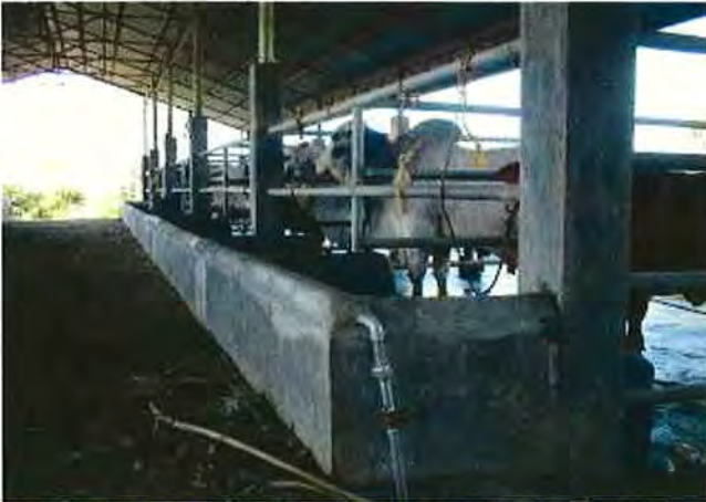
A new water supply line (pipe) to 5 watering troughs in a unit with one-valve control system is established
