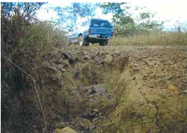
An eroded portion on the shoulder
