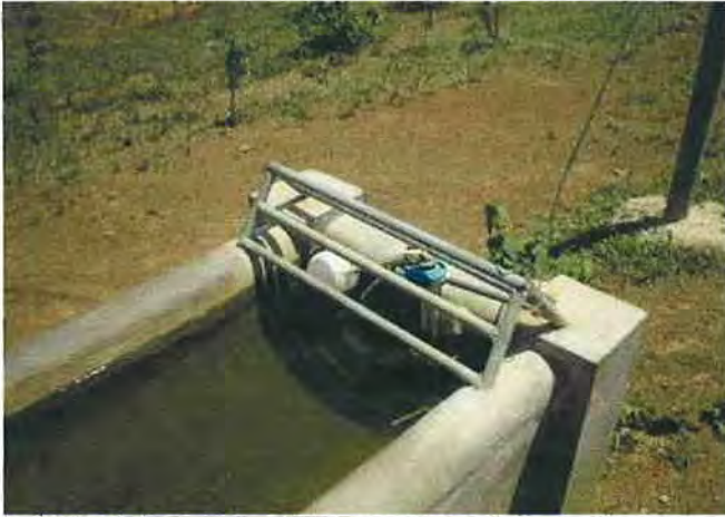
An automatic flow controller with its protector is installed to an unit
