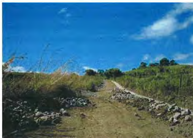
In the view of widening the road and establishment of a rip rap canal during the construction
