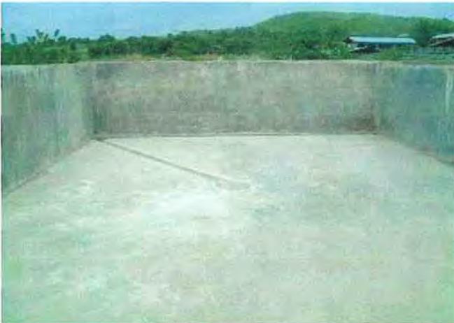
Alteration of floor, small catch basin and drainage for effluence from silage
