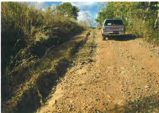
An eroded portion on the shoulder near the finish point of the road rehabilitation
