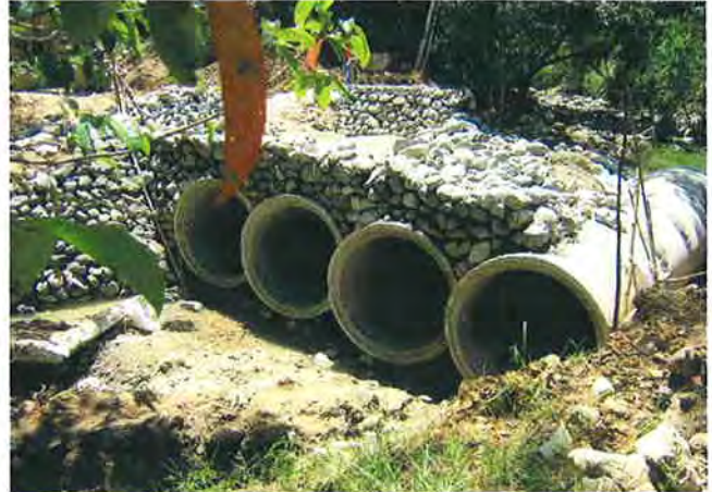
Four \phi 48 concrete barrels were installed with larger capacity instead of the box culvert
