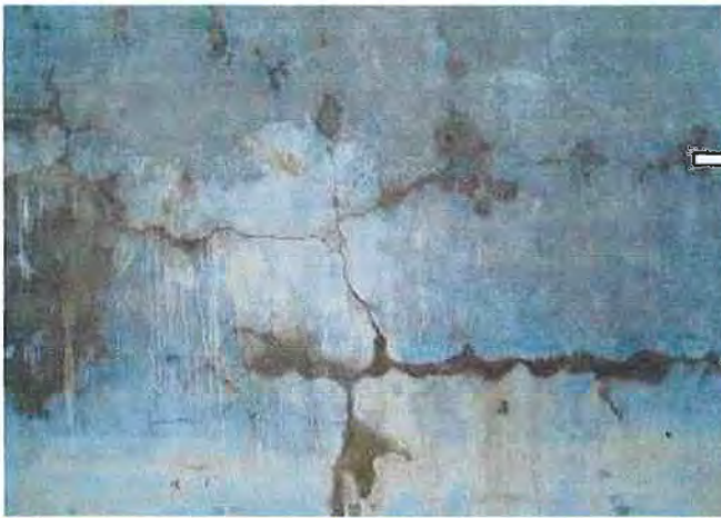
Cracks on the wall
