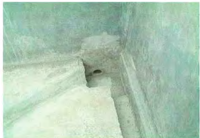
Drainage-end, catch basin and drain pipe
