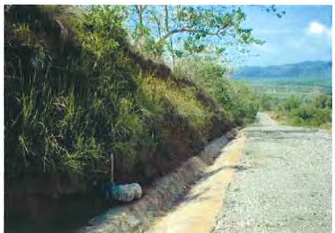
Covered with a large amount of soil and gravel
