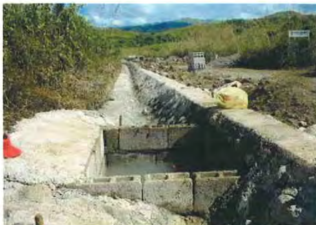
Open well near the junction of the simple access road. Actually, this is the catch basin of the water from the spring on the left side
