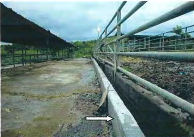
Receiving and draining mud and rain water from gate way to the weighing area
