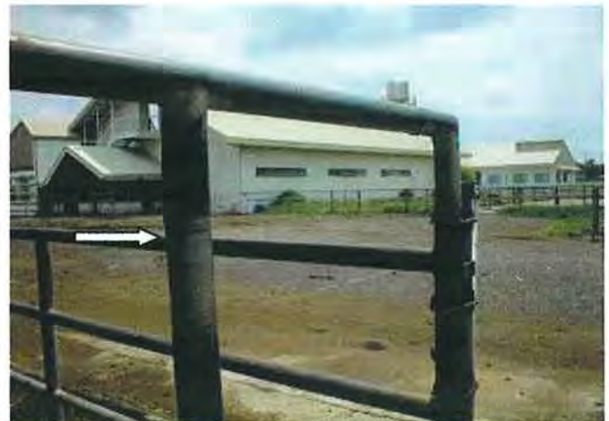
Pipes painted gray color were added
