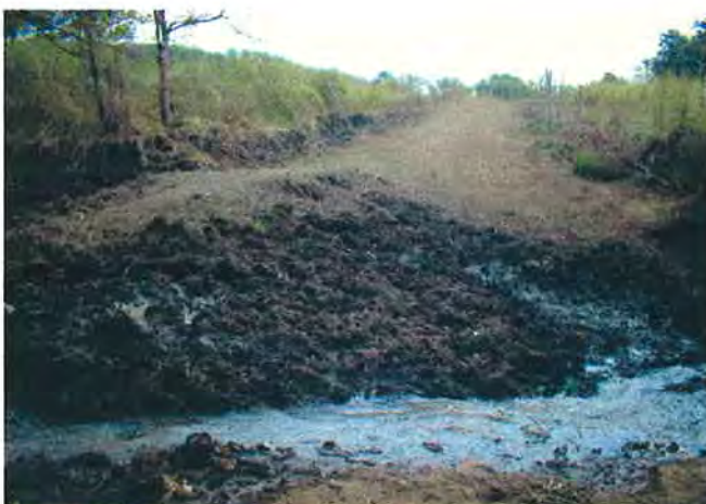
The worst portion of the road through a year
