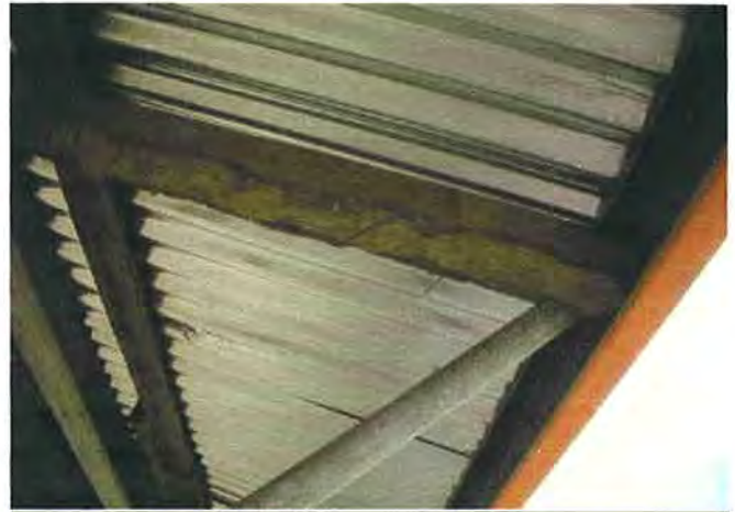
A wide view of re-roofing portion with painted frame with orange color
