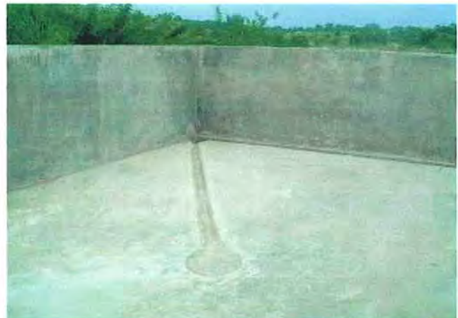
Alteration of floor, small catch basin and drainage for effluence from silage
