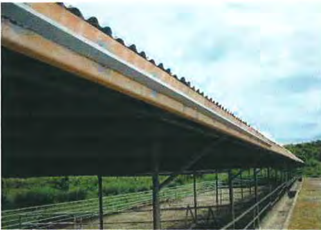
A L-angle bar was installed on the side to protect from damages of skid steer loader works
