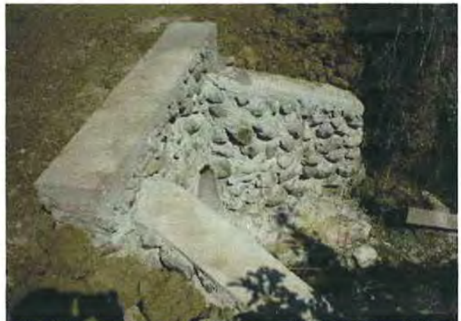
A big size of culvert with catch basin was prepared for draining water (Exit)
