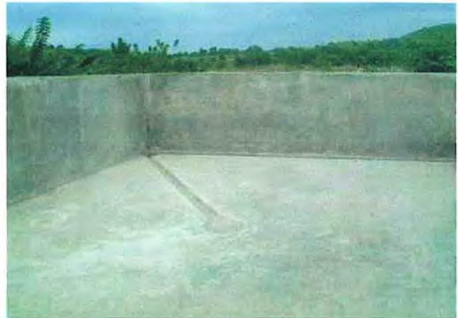
Alteration of floor, small catch basin and drainage for effluence from silage
